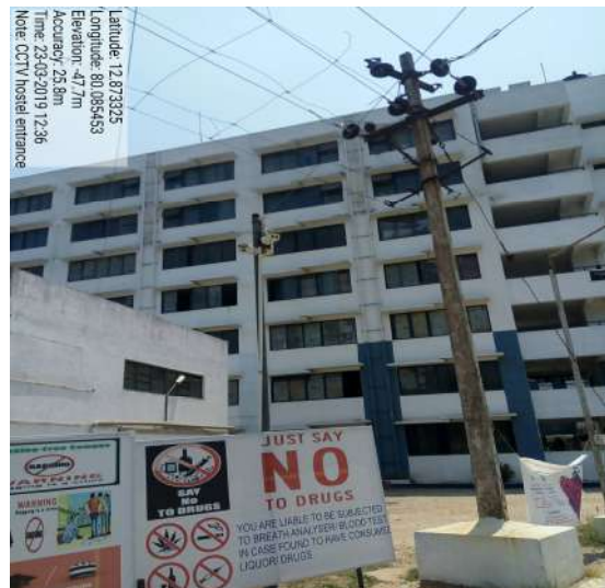
CCTV Camera installed at Boys Hostel Entrance
