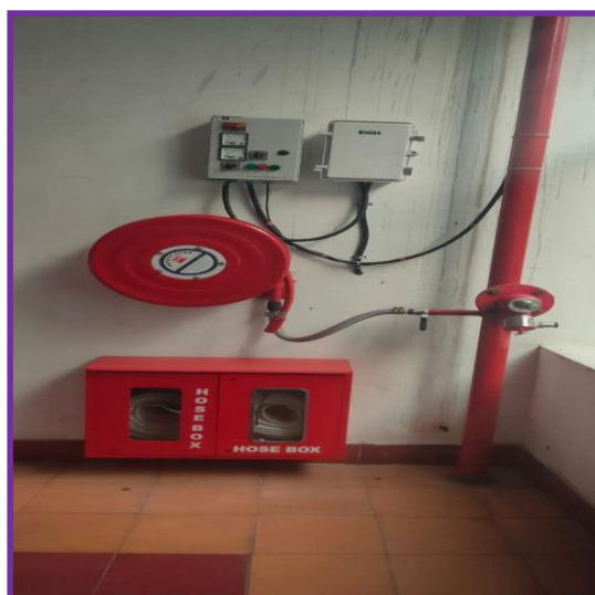
Sample Fire Extinguishers & First Aid Kit Placed in the College
