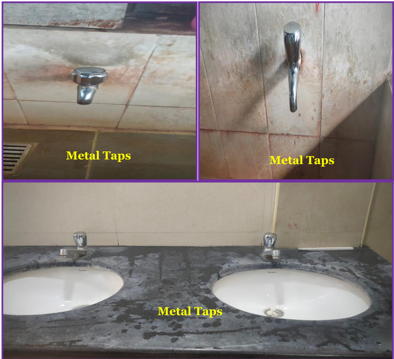
PVC and Metal Based Taping System for Water Distribution Line
