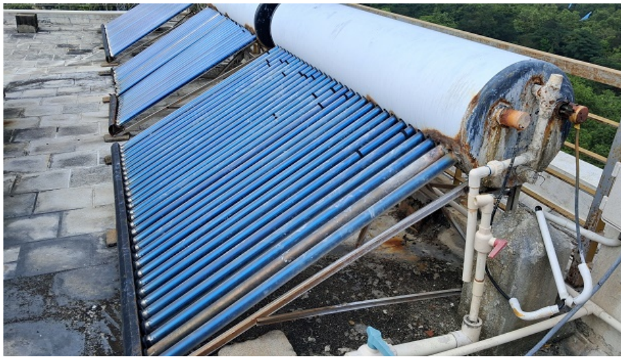
SOLAR WATER HEATER NOT IN SERVICE
