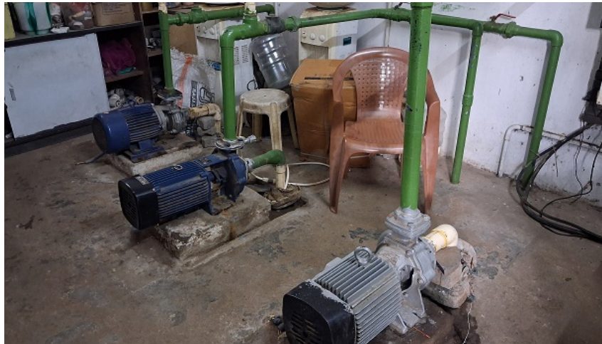
OLD WATER PUMPS
