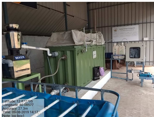
BIOBOX- Biogas generation unit
