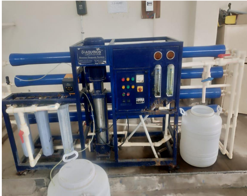
KBA MEN'S HOSTEL RO PLANT
