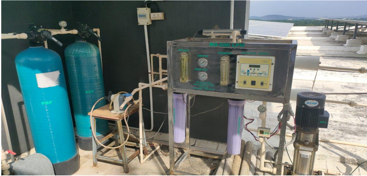
AERONAUTICAL BLOCK RO PLANT
